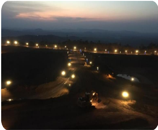
Main Haul road lighting in mines:
