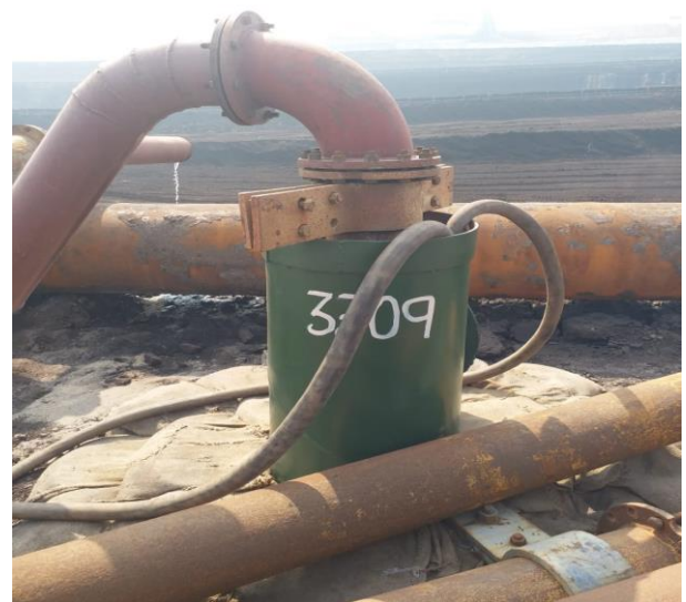
Fig 3.2: shows the pumping well no 3309 used for depressurizing the aquifer
